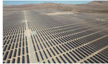
EDF PV plant in Atacama desert
